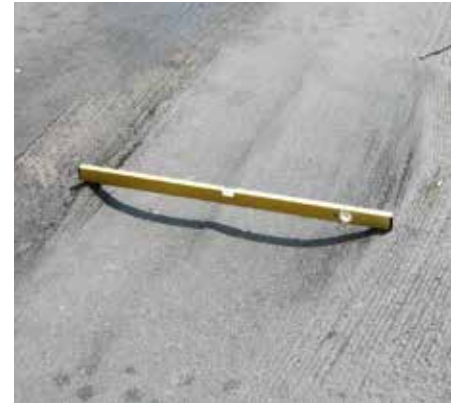
Rutting due to HGV traffic and higher axle loads
