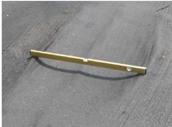
Rutting due to HGV traffic and higher axle loads
